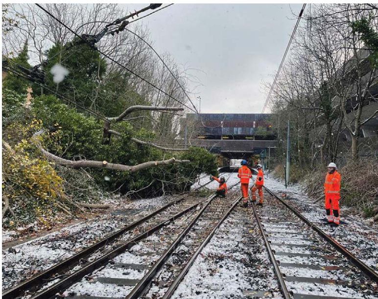
◀ Described as “the worst winter storm ever to hit the Metro”, Storm Arwen “savaged” the North-East in late November 2021 as 145km/h (90mph) gales felled trees and tore down overhead lines across the network. Amazingly, the trains were up and running again in less than 48 hours.
