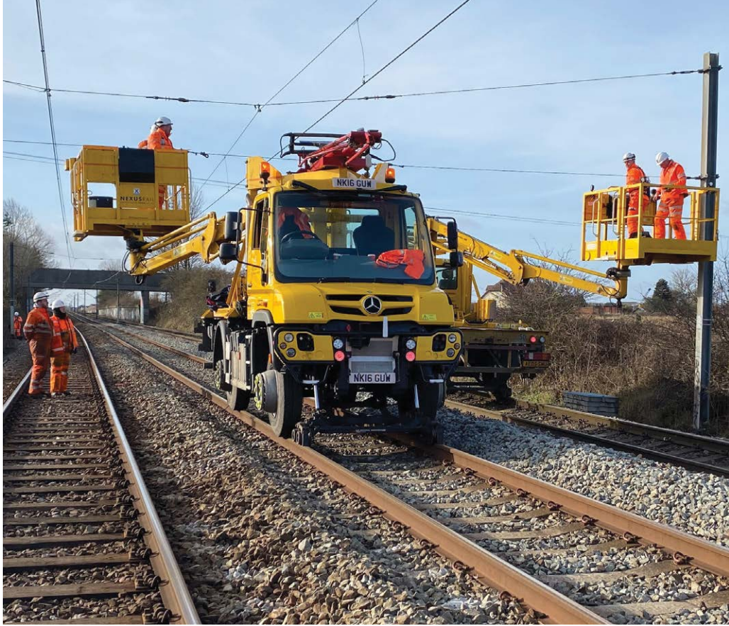
▲ Over the past 12 years the Nexus Rail engineering team has renewed track, structures, electrification, and modernised the original Tyneside network to future-proof the Metro and prepare for the new fleet.
