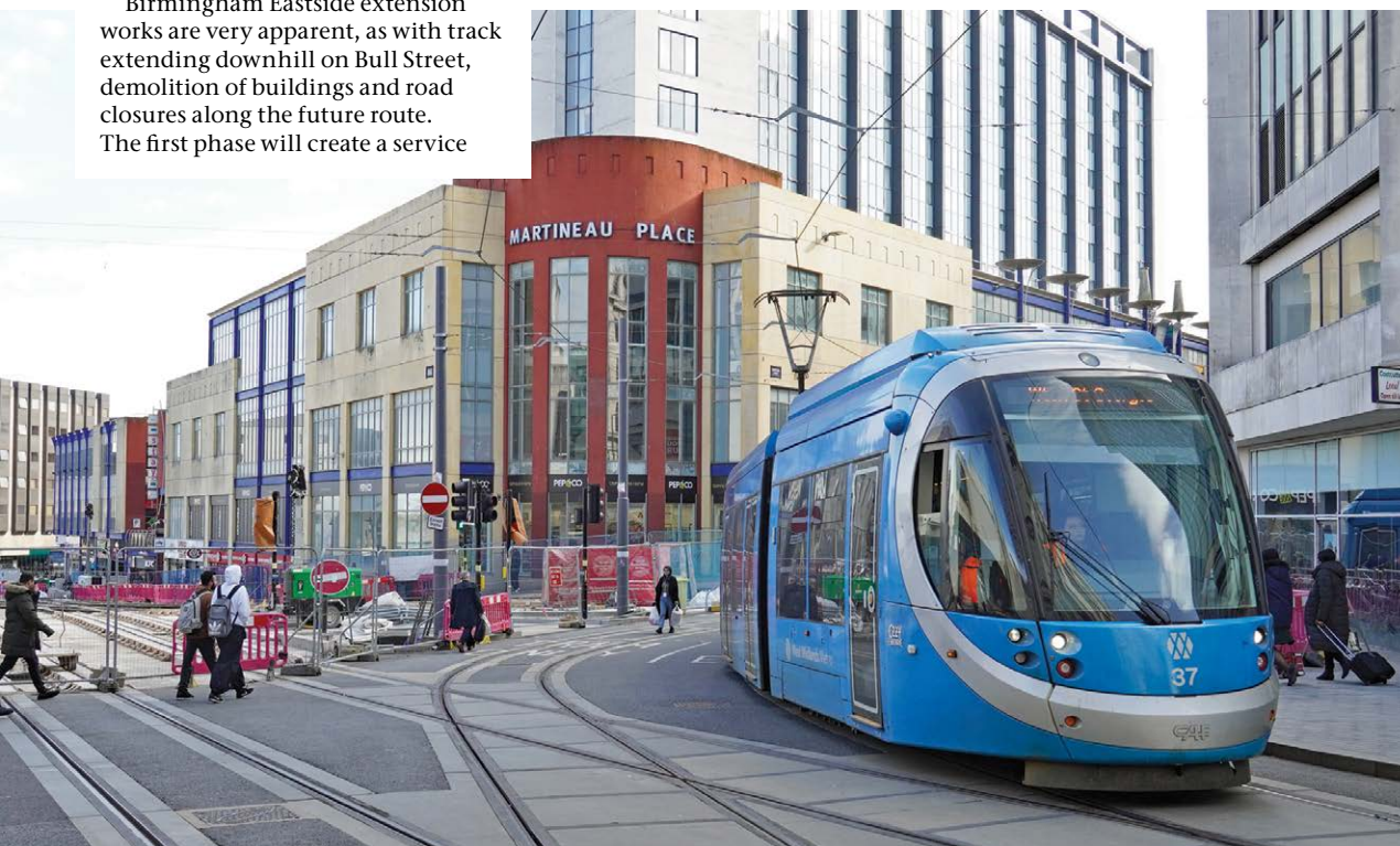
◀ LEFT: A junction for the Birmingham Eastside extension has been installed at the intersection of Bull Street and Corporation Street.
