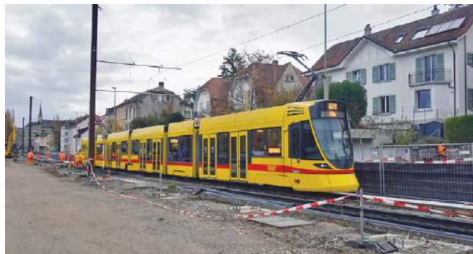
▲ ABOVE: A BLT Stadler tram on the temporary single-track alignment. In the foreground is the area once occupied by now demolished houses. A. Thompson
