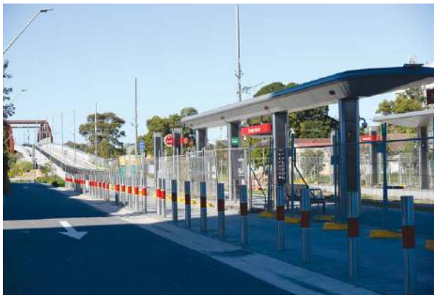
▲ ABOVE: The 12km Parramatta line under construction - a project that has cost the NSW government AUD3.5bn and is set to launch this year.
