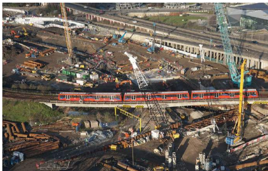
▲ ABOVE: A key part of early area redevelopment on the Woolwich Arsenal line near Royal Victoria Dock in January 2023. Neil Pulling
