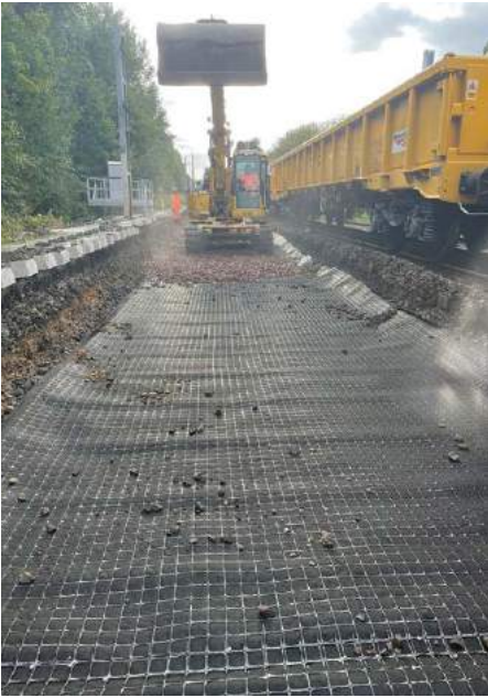
▲ ABOVE: The new track formation being laid east of Hebburn Metro Station. Nexus
