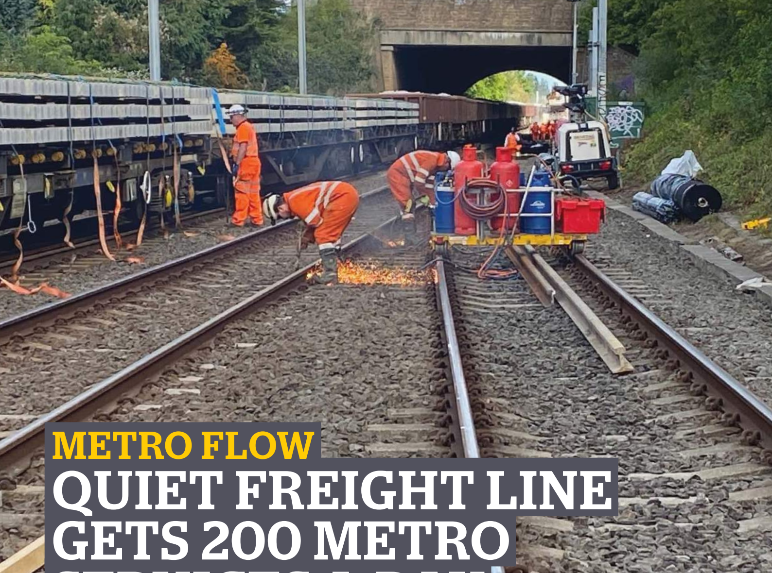
▲ ABOVE: Track work takes place at Victoria Road bridge, Bill Quay, during Metro Flow construction work in autumn 2022. Nexus
