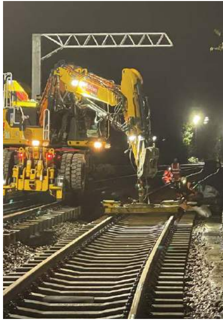
▲ ABOVE: New track installation on the outbound line at Hebburn Platform 2. Nexus
