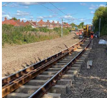
◀ LEFT: New track installation immediately east of the Pelaw Junction Inbound Cord. Nexus
